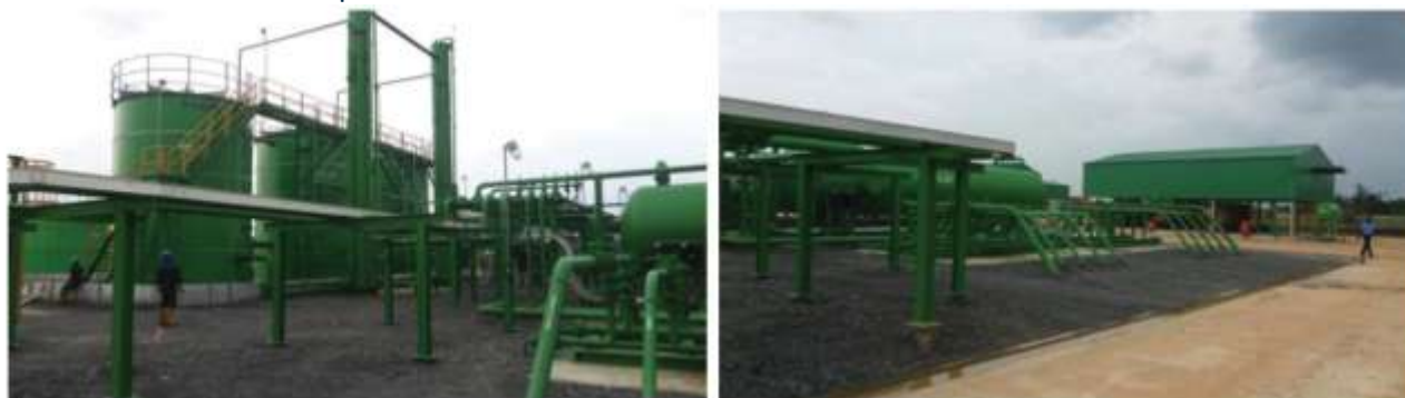
Exhibit 3: Oza field infrastructure - new production facilities
